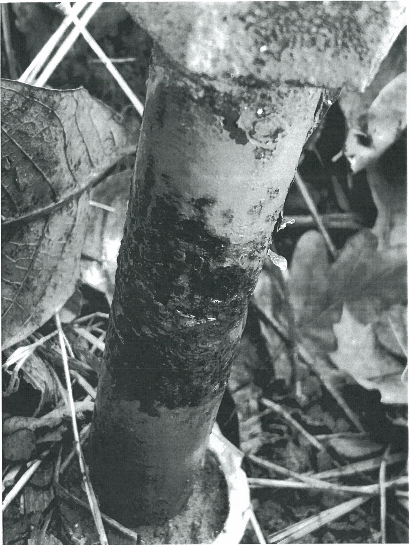
Photo #3, 1/17/19, 3115 Farmway Rd. Caldwell, ID. Hpss 07676-317. Outlet line below valve is pitted. Photo taken by Inspector Russo at 12:17 PM.
