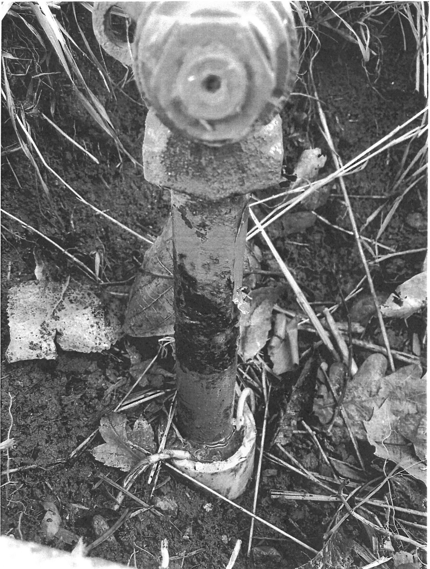
Photo #2, 1/17/19, 3115 Farmway Rd. Caldwell, ID. Hps 07676-317. Outlet line below valve is pitted. Photo taken by Inspector Russo at 12:15 PM.
