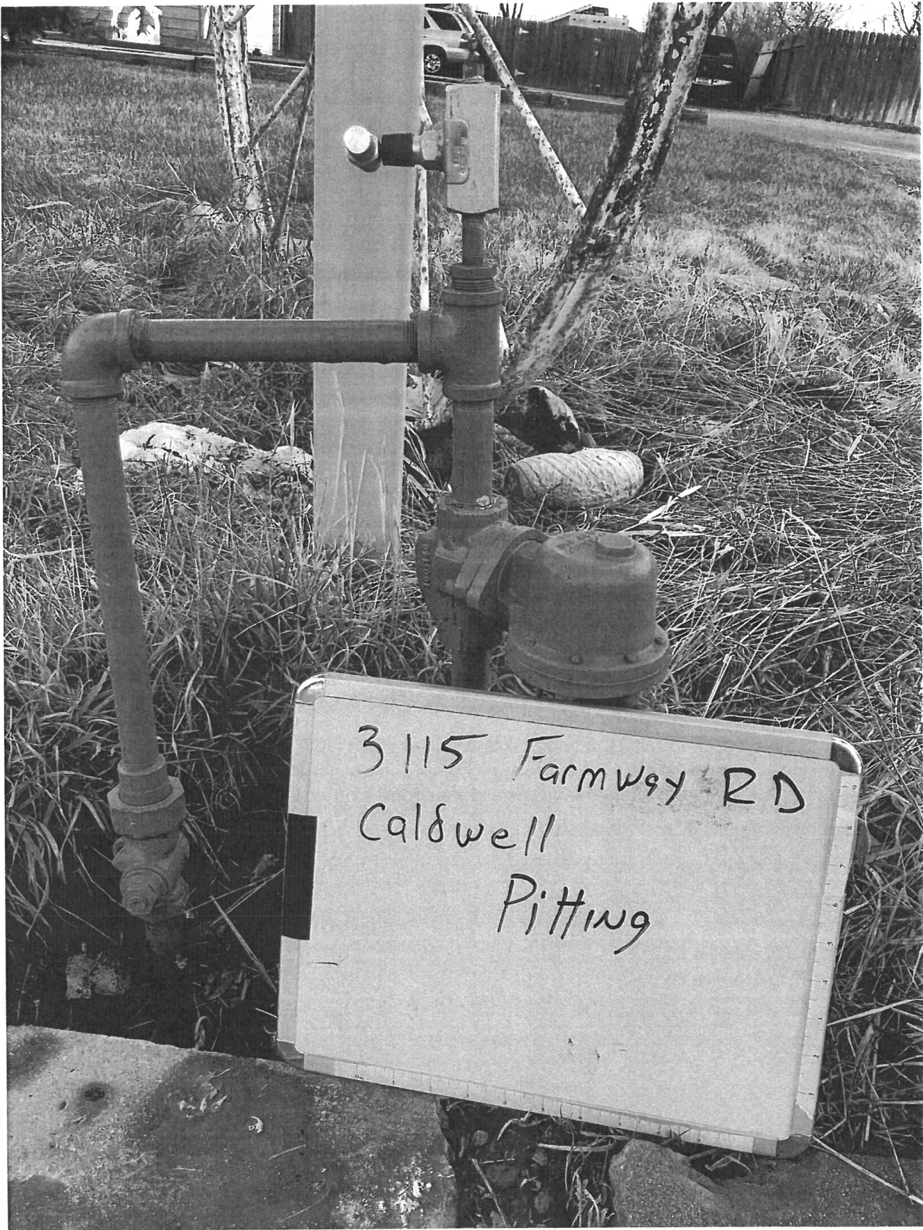
Photo #1, 1/17/19, 3115 Farmway Rd. Caldwell, ID. Hps 07676-317. Outlet line below valve is pitted. Photo taken by Inspector Russo at 12:17 PM.
